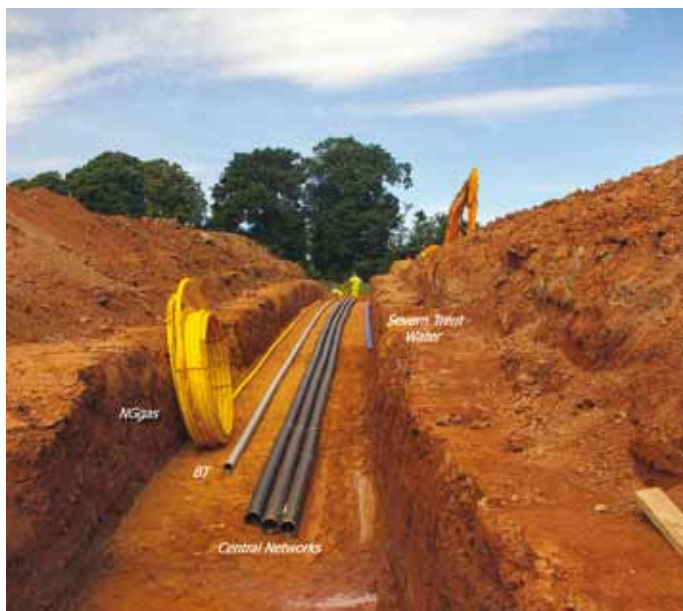
A46 Newark to Widmerpool Improvement Syerston Services Crossing Balfour Beatty Innovation: Combined Services Trench by North Midland Construction PLC, giving programme and safety benefits
